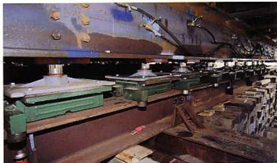
FOR LIFT AND SUPPORT: The roller beams (below) and the jacking beam (above) await action on a crib at the old site.
